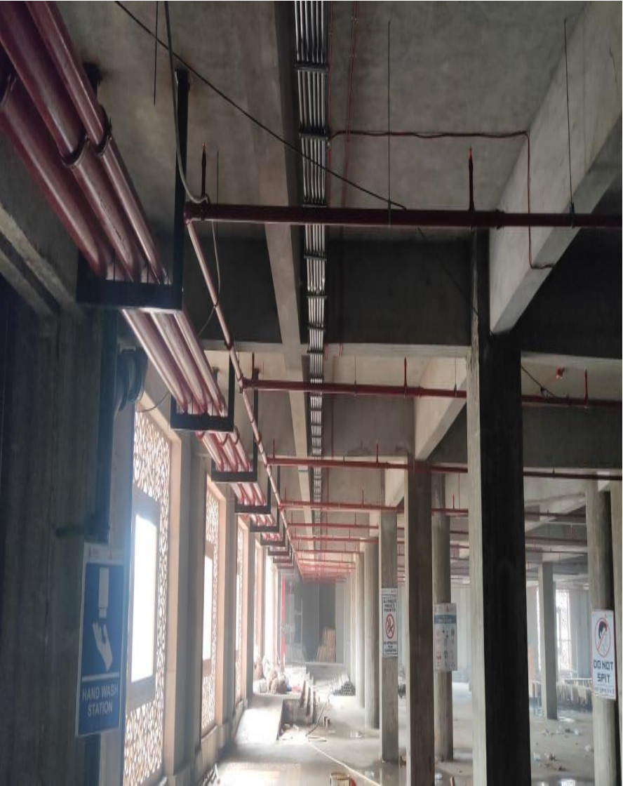
ACCESS CONDUIT – UTILITY FLOOR
